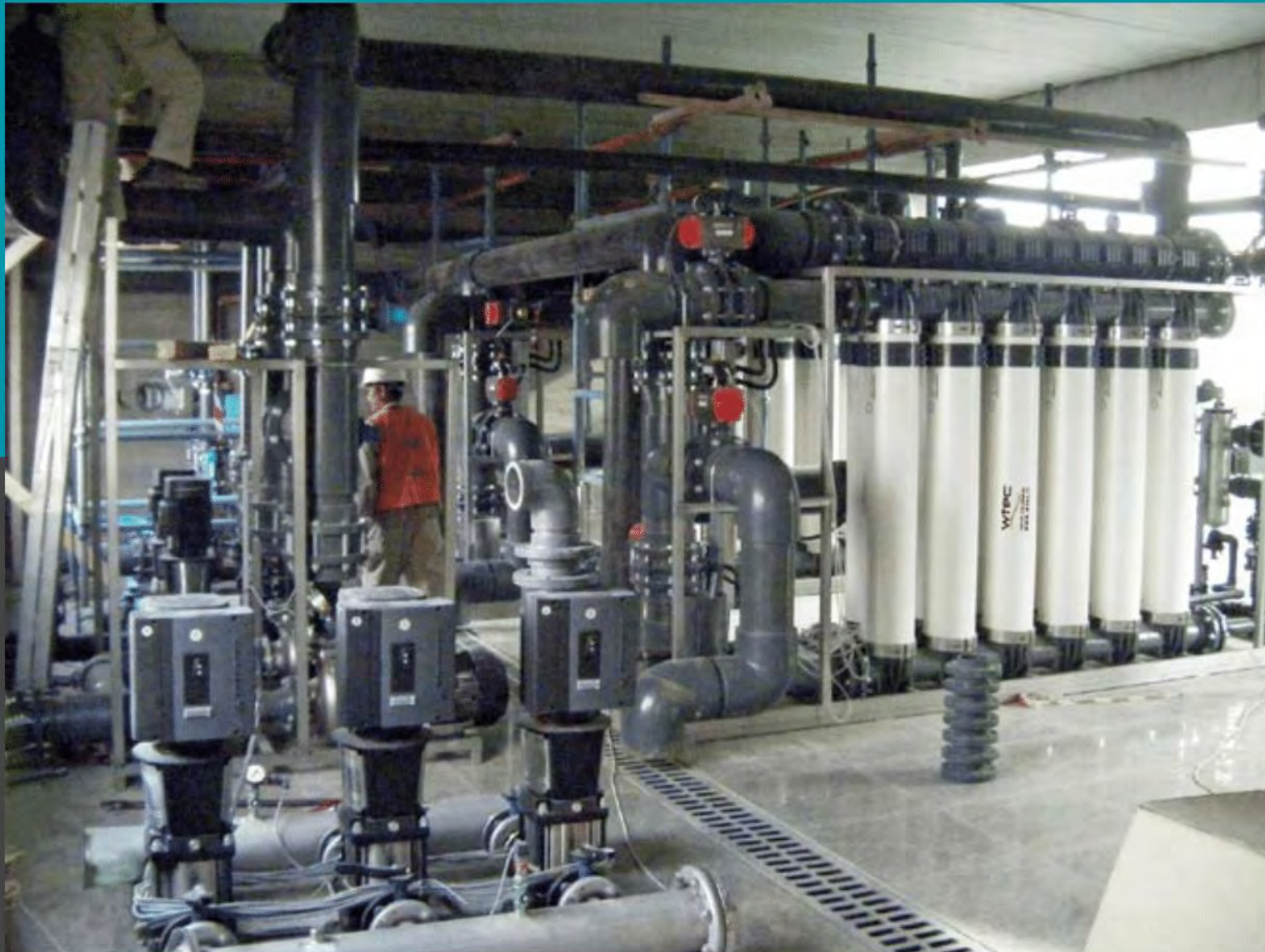
Ultrafiltration plant with hollow fiber membranes in PES - Flow 2x40 mc/h, Wastewater refining and reuse
