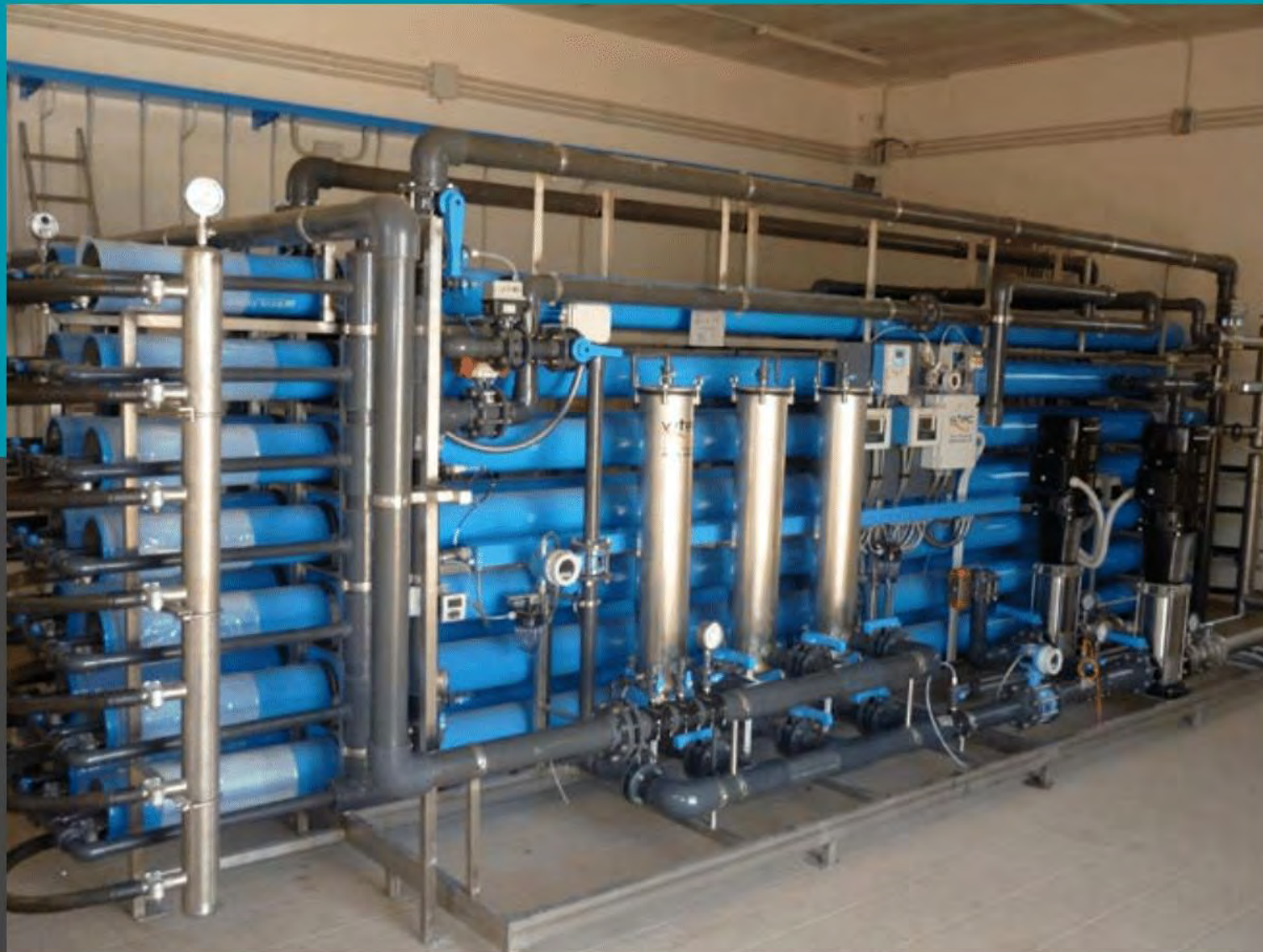
Reverse osmosis plant BWP 1320 Mod. - Flow 2x55 mc/h, Potabilization plant
